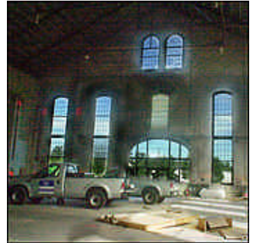
Workers begin construction on the Arsenal Center for the Arts, with a spring opening planned. - STAFF PHOTO BY KEITH E. JACOBSON
